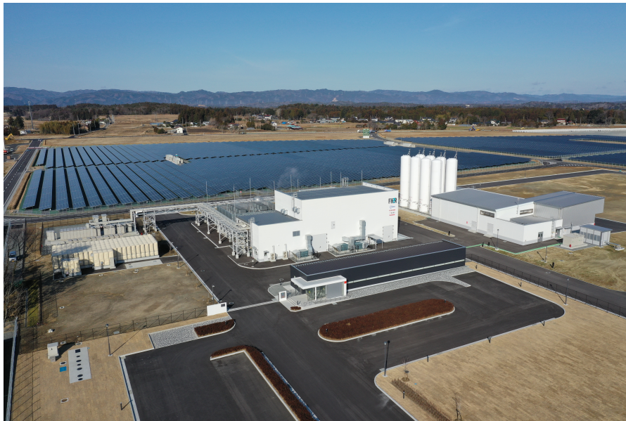
Figure 1.2: A 10 MW PV-Electrolysis plant in Fukushima, Japan [14]
