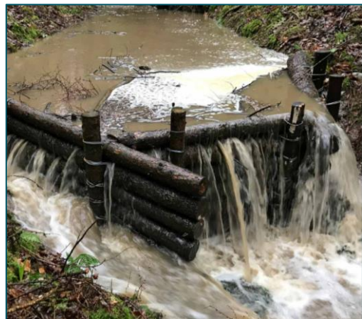
Figure 4.7 – Leaky barrier at Flimby, England (Bridges et al., 2021b).
