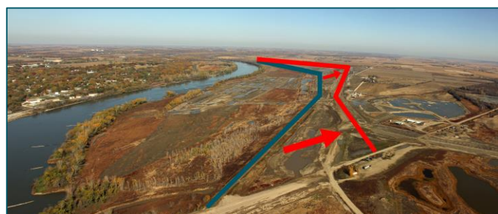
Figure 5.10 – Missouri River Levee Unit L-575 'HWY-2' Setback under construction in October, 2012 (Crane, 2012).
