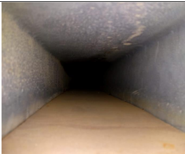
Figure F7: Inside of pipe. Fixed sand bed on bottom wall
