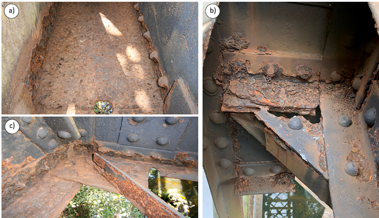
Fig. 3. Detail of corroded elements in the Paraíso bridge a) chord web b) gusset plates at the connection between stringers and cross-girders c) connection of the lower lateral bracings to the chords.
