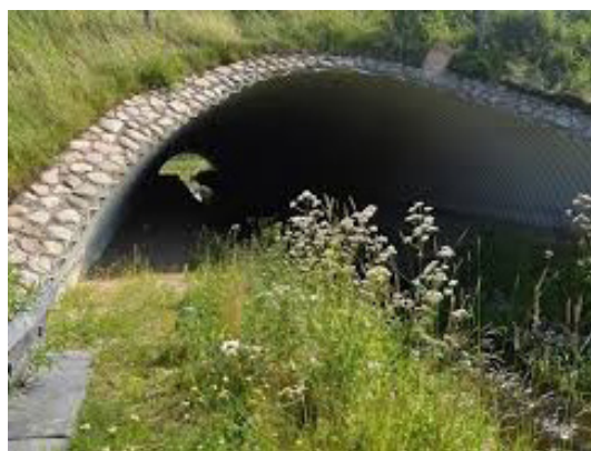
Figure 8.43: Culvert that also allows small animals to cross ( Petero_dk, n.d. )
