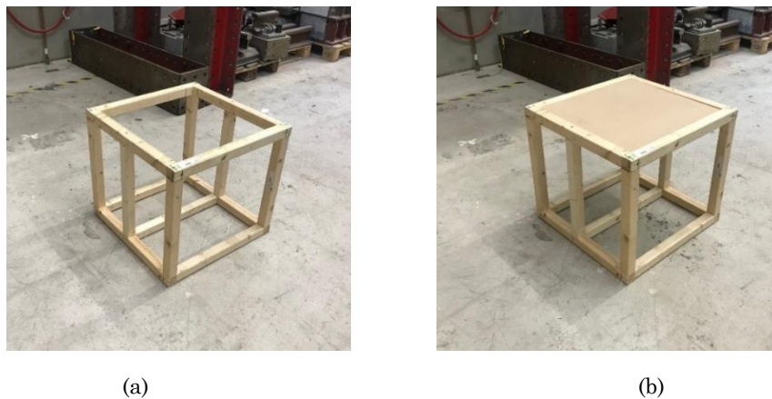
Figure 6.2: The base of the formwork: (a) external timber frame; (b) precisely cut plywood plate that fits in the opening.
