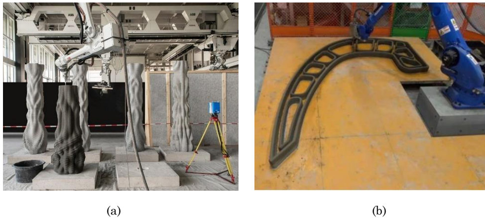
Figure 2.12: Extruded concrete 3D printing for different implementations: (a) tailor-shaped columns; (b) cantilevering shell structure (photo credit: (a) Axel Crettenand; (b) (Sakagami et al., 2020)).
