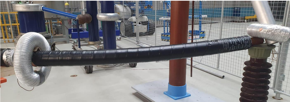
Figure 32. Photo of one of the temporal terminations at the HVDC cable.
