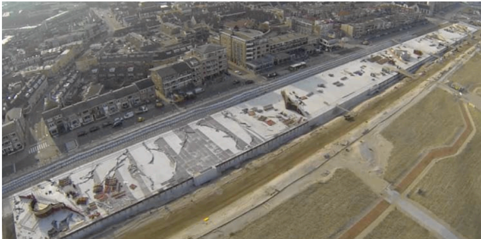
Figure 73 The concrete parking garage still uncovered by sand during construction Source: [The Parking Garage Under Construction] (n.d.)
