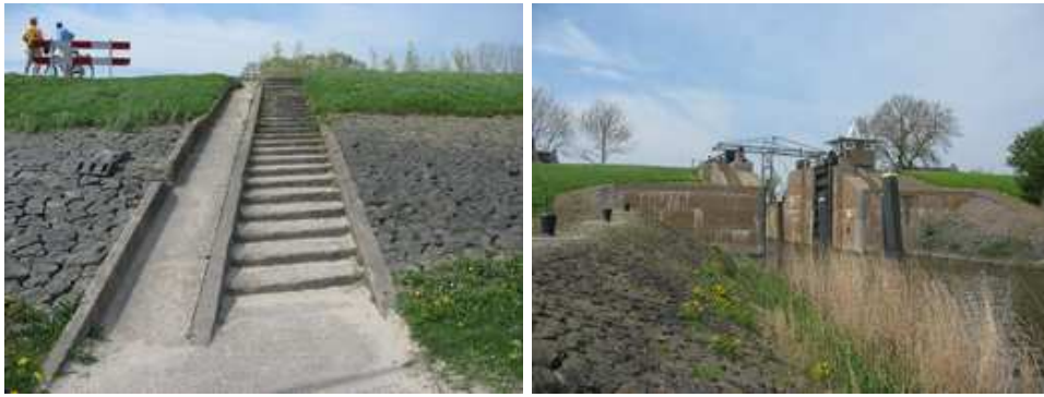
Fig. 4.23. More PS targets in the Netherlands: (left) dike covered with basalt blocks that is a distributed PS, (right) sluice that is most likely represented by a multi-bounce reflection.
