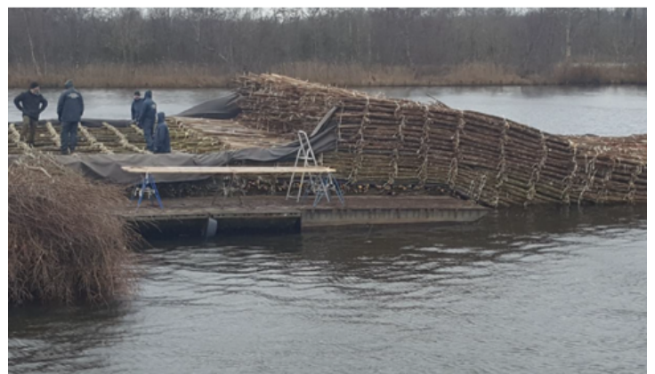
(b) Brushwood groyne of layered fascine mattresses (collection Van Aalsburg BV)
