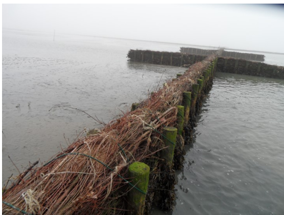
(a) Sheet pile groyne filled with coniferous branches at a salt marsh in the Wadden Sea (collection Van Aalsburg BV)
