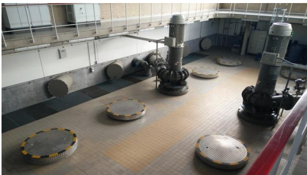
Figure 28: Pumps 1 and 3 (own image)
