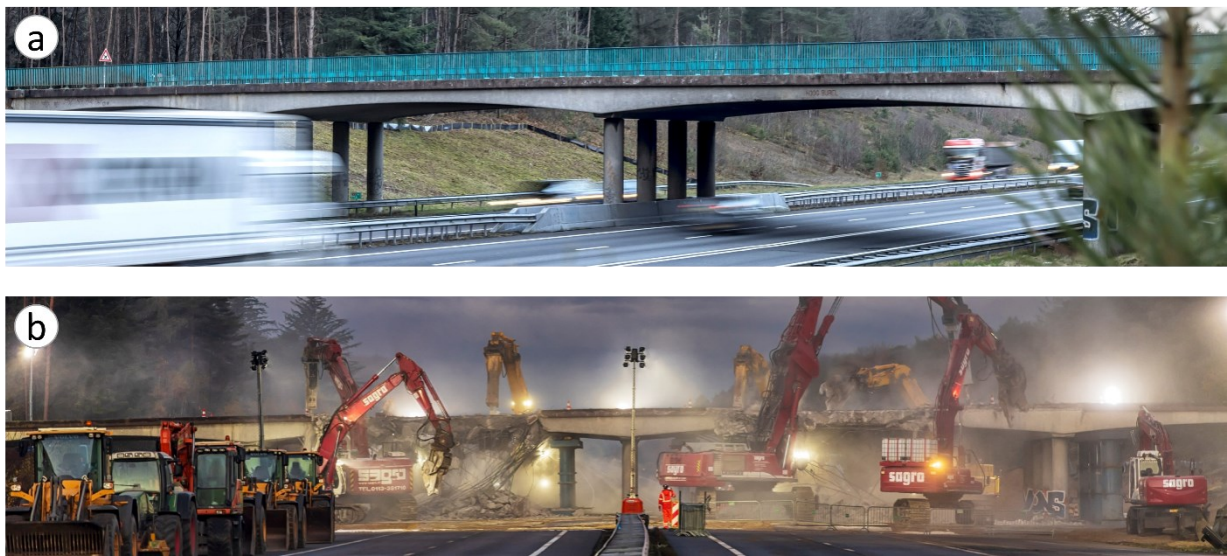
Fig. 1. Demolition of Hoog Burel viaduct (A1), the Netherlands: a) before demolition, b) during demolition (November 2022). Credits go to Rijkswaterstaat [10]
