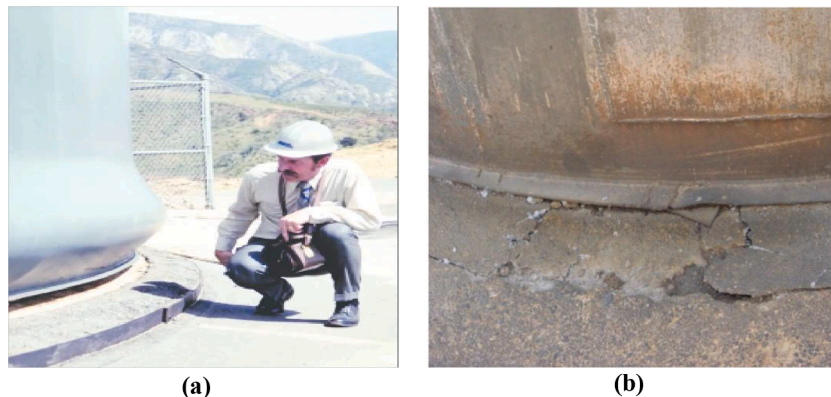
Fig. 3. Elephant-foot buckling and cracked foundation of steel tanks, (a) Elephant-foot buckling of a tank wall (courtesy of University of California at Berkeley) [38]; (b) Cracked foundation of the tank during the Silakhor Earthquake of 2006 in Iran [34].
