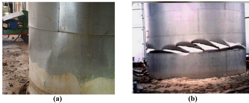
Fig. 2. Diamond-shaped buckling of steel tanks, (a) Diamond-shaped buckling of a steel tank during the Silakhor Earthquake of 2006 in Iran [36]; (b) Diamond-shape buckle of a steel tank in Kobe at the 1995 Kobe Earthquake [37].
