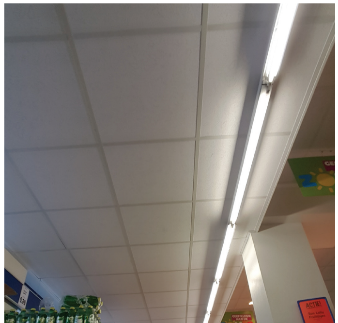
Fig. 103 Fig. 54: Drop ceiling, Lidl Doctor H.J. van Mooklaan Rijswijk (source: own image)
