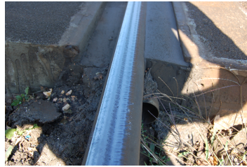
Figure 20 Asymmetric ground rail profile (location: Woeziksestraat Ht-Nm, 59.026; time: 23/08/2016) (ProRail, 2018a)
