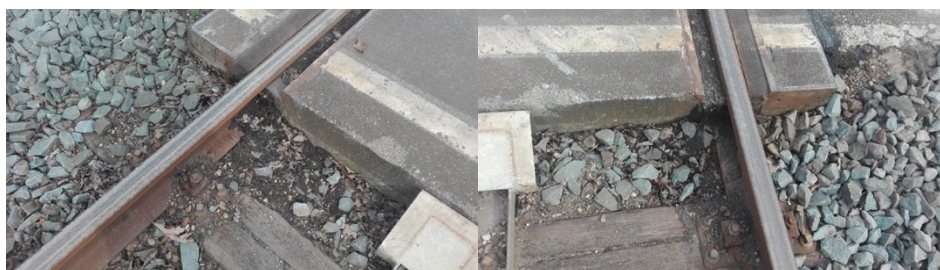
Figure 13 Wooden sleepers in the transition and pollution at the rail ends (ProRail, 2018a)
