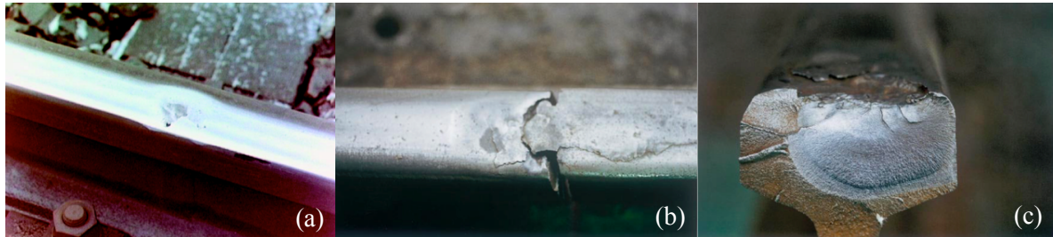
Figure 9 (a) Appearance of squats; (b) Rail fracture resulting from squats; (c) Cross section of the broken rail (UIC, 2002)
