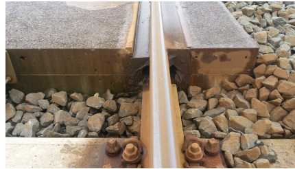
Figure 11 The end of Harmelen LCS / connecting area to the ballasted track (location: IJsseldijk 92.673; time: 17/09/2015) (ProRail, 2018a)
