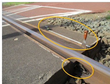
Figure 15 Corkelast® not completely attached to the channel wall & possibly corroded area (location: Almelosestraat, 19.373; time: 01/08/2016) (ProRail, 2018a)
