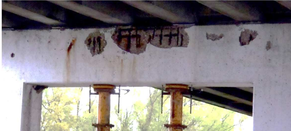
Figure 3-16: Corrosion and spalling of a supporting beam from the Nijkerkerbrug, a RC bridge in the Netherlands.
