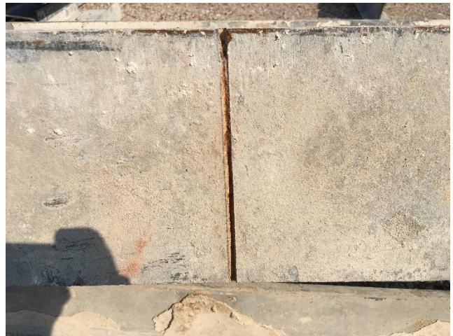
Figure 8: damaged donor steel after disassembly
