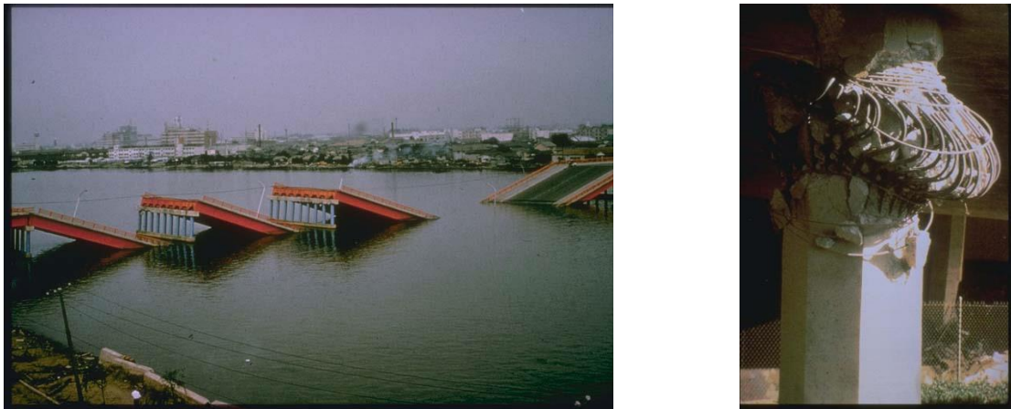
Figure 2. Unseating of bridge deck (left). Shear failure due to insufficient detailing (Courtesy of NOAA/NGDC)
