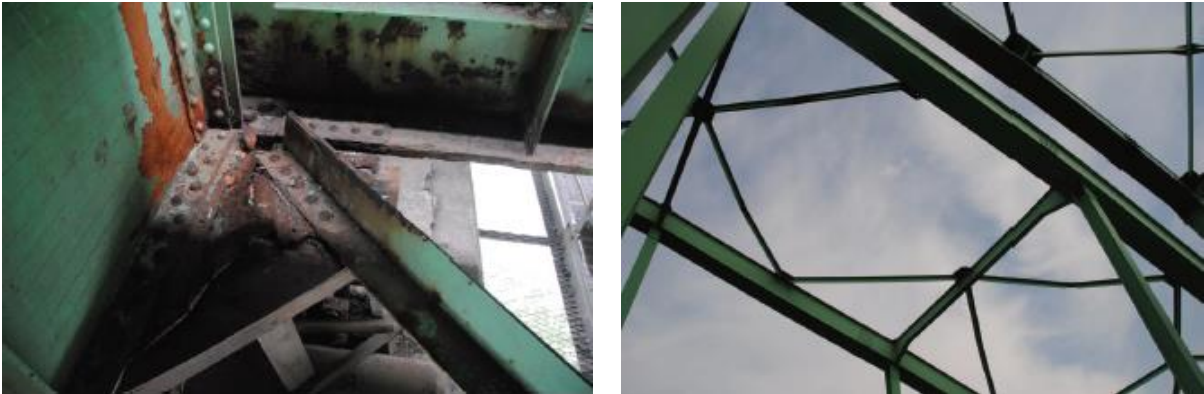
Figure 3. Disconnection and buckling of braces. Tennoh Bridge. Japan (Kawashima K (2012))
