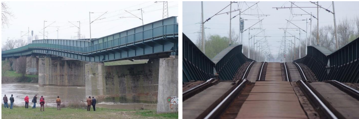
Figure 1. Scour around a rail bridge over the River Sava, Zagreb (picture courtesy of Croatian Railways 2009)
