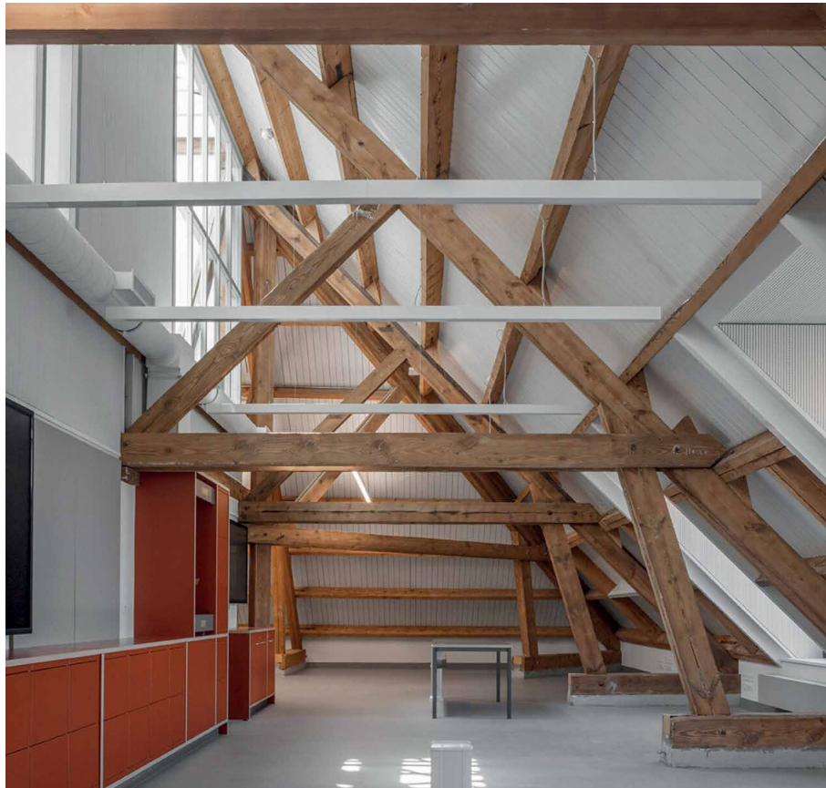
FIG. 4.10 Attic trusses at the old building of the Campus Cadix. Source: KSA
