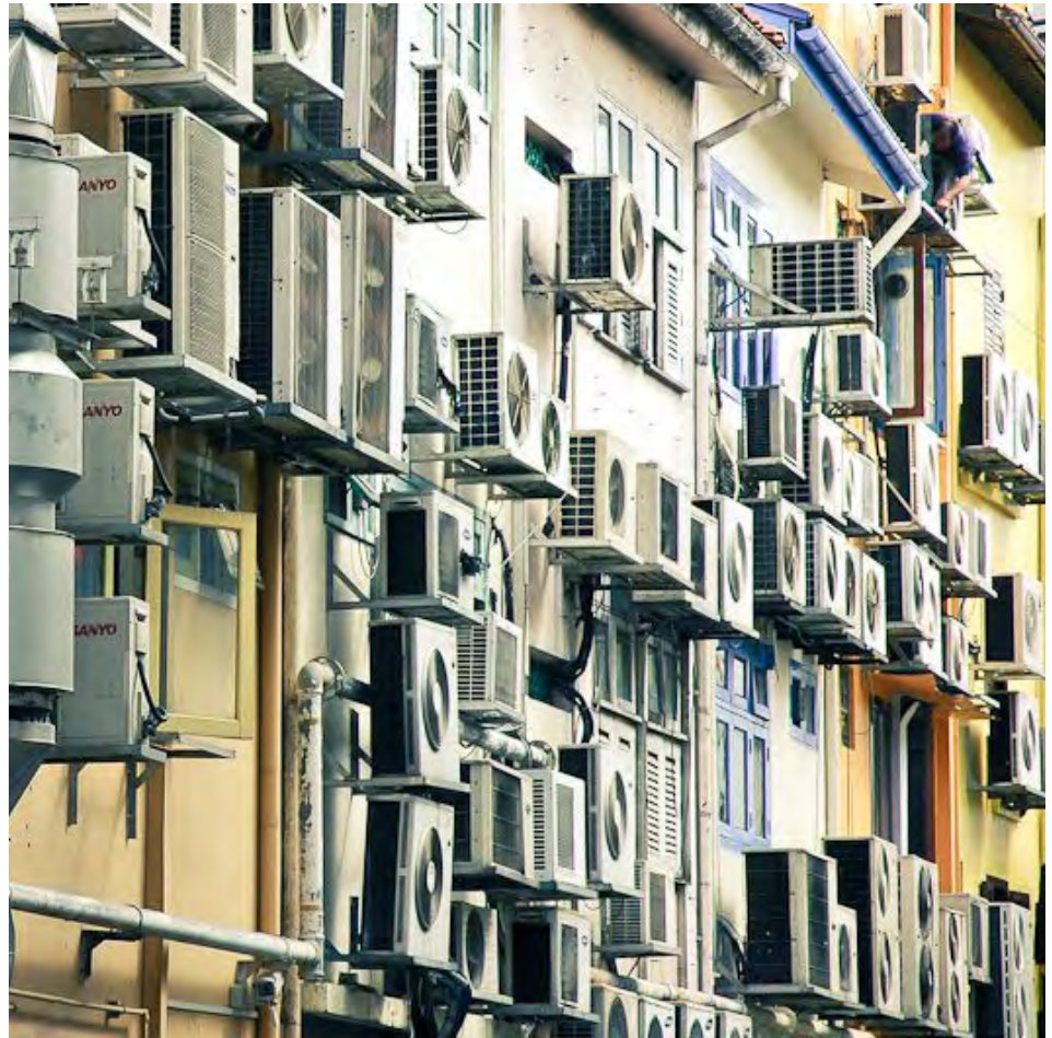
Figure 4-1 : A normal scene of CDU units of split type air-conditioned system in tropical countries
