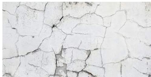
Figure 9.3: Map cracking (123 rf, 2018)
