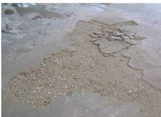
Figure 2.1: Delamination (CoGRlpedia, n.d.)
