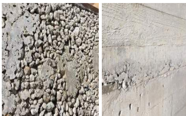
Figure 1.1: Honeycombs (ConRep concrete repairs, n.d.) (Patricia, 2016)
