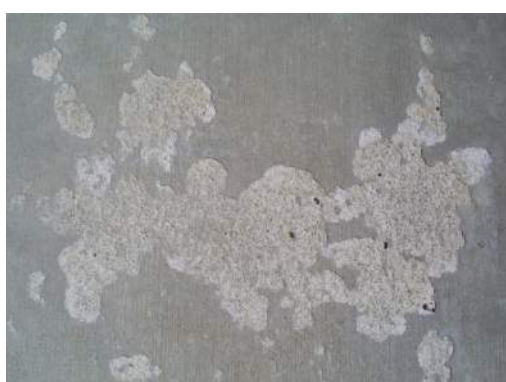
Figure 3.2: Scaling (Power line usa, n.d.)
