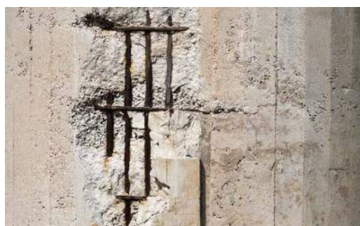
Figure 4.1: Spalling due to corrosion (JHA Australia, n.d)
