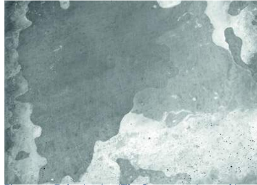
Figure 8.1: Delamination (The Concrete society, n.d.)
