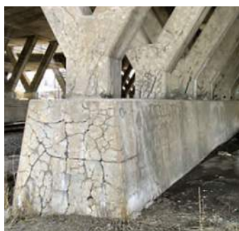
Figure 9.1: Map cracking (Hess, n.d)
