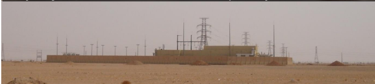
Electrical grids and the power sub-station of University of Hafr Al Batin, eastern part of the KSA
