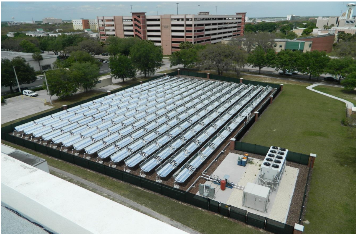
Figure 5.19: Thermal energy storage system (USF Student Green Energy Fund 2016, 1)
