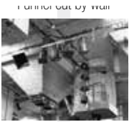
Stuff on the ceiling
