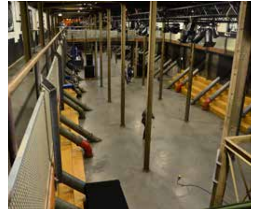
Pipe system that leads the grain from the distribution floor to the silo bins
