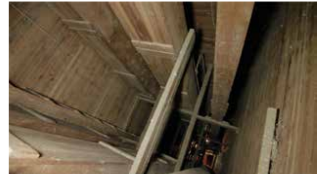
Inside of a wooden silo where the elevator leg is visible ( http://www.sandpointfilmmakers.net/filmmaking/co-op-grain-elevator-sandpoint-idaho/ )
