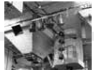
Stuff on the ceiling
