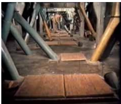
5. The distribution floor with the pipes that let the grain into the silos
