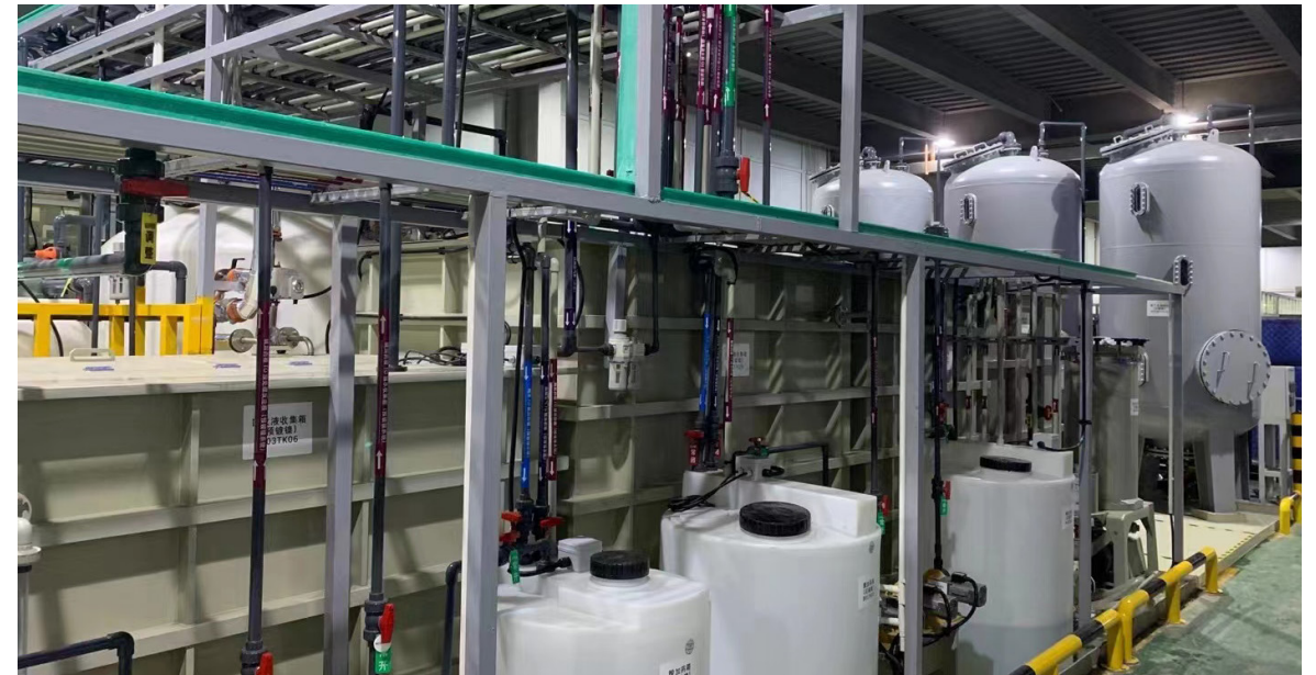
Photo source: Electroplating Nickel Resource Reuse centre, Shanghai Shunfan Environmental Protection Technology Co., Ltd., https://www.12345ep.com/product-item-12.html
