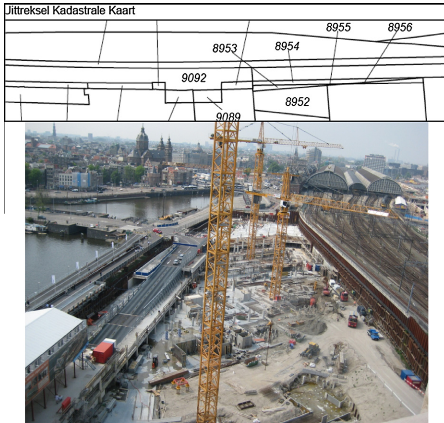
Fig. 10. Fragmented parcel pattern (area covers appr 10 \times 45 m) established for several physical objects required in the construction phase of a building complex.
