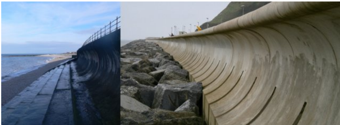
Figure 1.4: Left panel: Wave return wall located in Penrhyn Bay, Great Britain. Right panel: Recurved seawall at Scarborough. Image taken from Castellino et al. (2019)
