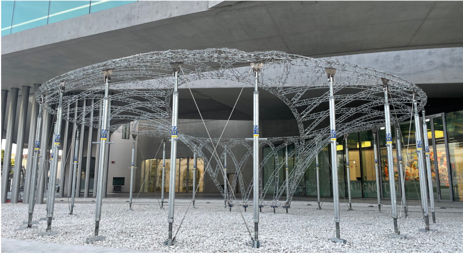
Fig. 10. Demonstrator in the construction stage of the completed gridshell made of bending-active splines.
