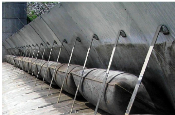
Figure F.2: Example of gate system with an inflatable bladder (Daniel & Paulus, 2018)
