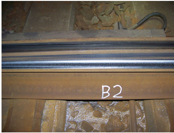
Figure 14. Switch panel of ‘severely’ wearing switch (left switch and stock rail). Wear debris present, high roughness of gauge face. No lubrication marks.
