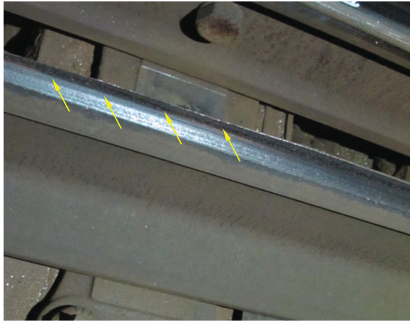
Figure 12. Severely worn switch rail (inspection December 2014).
