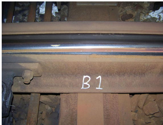
Figure 15. Switch panel of ‘mild’ wearing switch (left switch and stock rail). No wear debris observed. At the gauge face remains of lubrication are present.
