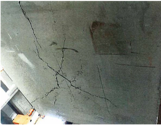
FIGURE 21 Crack pattern at bottom of slab P-3 (with fibers and ties) after the test
