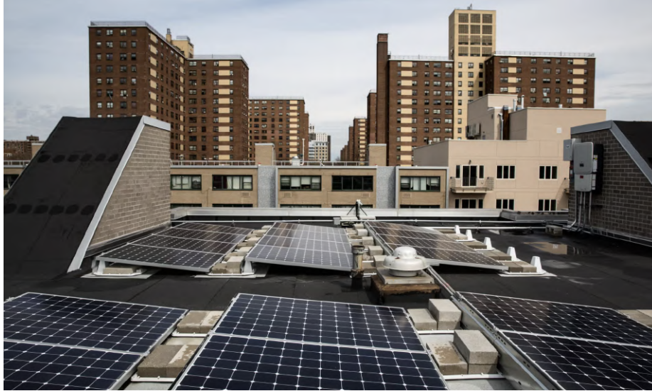
Figure 4: Rooftop Example inside the Brooklyn Microgrid [17]
