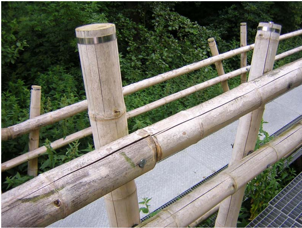
Figure 20: Cracking of bamboo culm when directly exposed to climatic conditions
