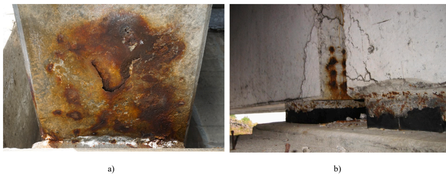
Fig. 30. Corrosion cracking in bottom of pretensioned girders: a) significant corrosion cracking in the NIB girder bottom flange near support, bridge close to Kristiansund; and b) corrosion cracking and spalling in the NIB girder-ends, photo by NPRA [7].
