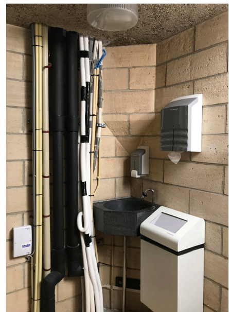
Fig 12: Photo of installations
