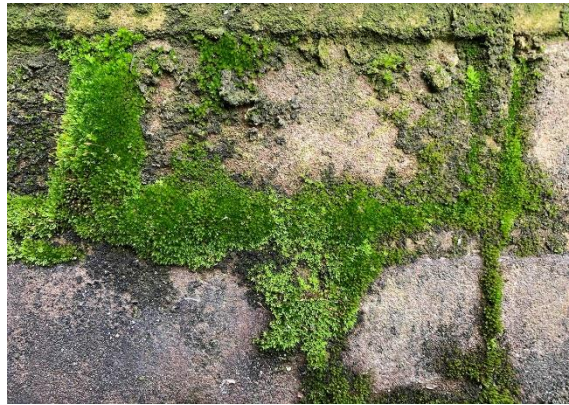
Figure 1. Natural moss growth on masonry.
