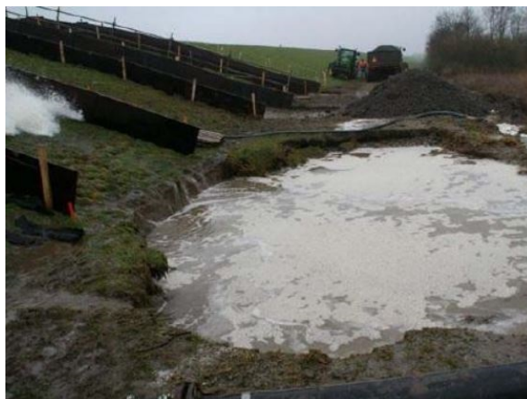
(b) Jet erosion at the toe of the dike
