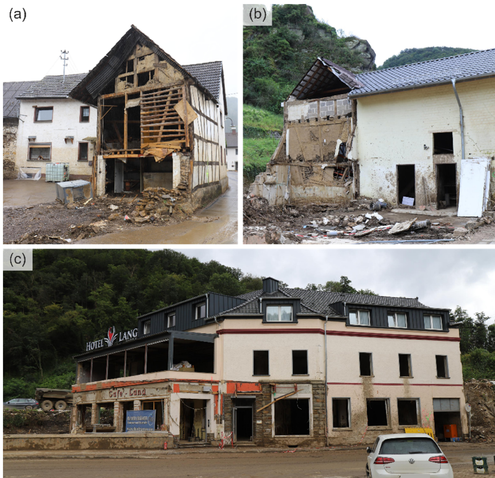
FIGURE 10 Failure of traditional half-timbered structures due to flood loading in Schuld (a) and in Kreuzberg (b) while (c) shows a modern construction in Altenahr, with a concrete structure that sustained flood loading.
