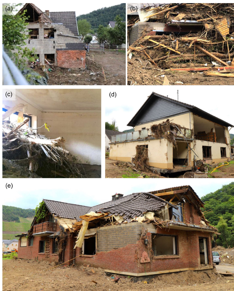
FIGURE 15 Photographs of remains of debris-dams accumulated at buildings. (a) Insul; (b, c, e) Dernau (same building); (d) Brück.
