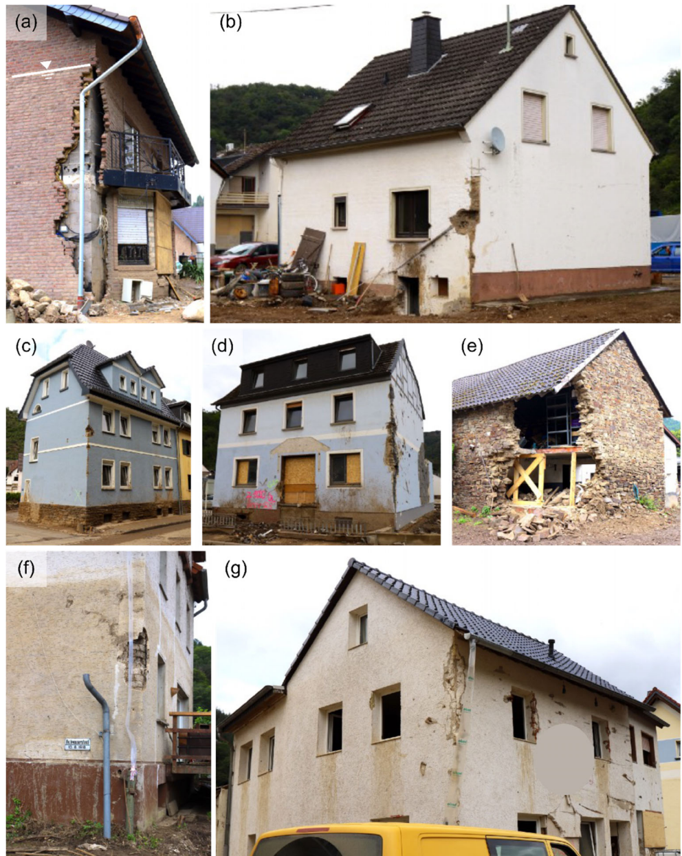
FIGURE 14 Damage and partial failures caused by the impact of floating debris, below the water-mark. (a) Dernau; (b) Altenahr; (c, d) Kreuzberg; (e) Schuld; (f) Brück; (g) Kreuzberg.
