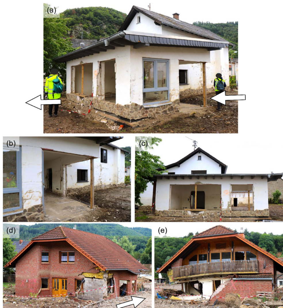
FIGURE 17 Building damage associated with the failure of single elements: (a–c) failure of a pillar in Schuld, likely associated with the debris reported inside the structure (removed, hence not visible in the picture); (d) wall tilting forward and (e) column missing at the corner in Insul. Red arrows indicate the suspected flow direction.
