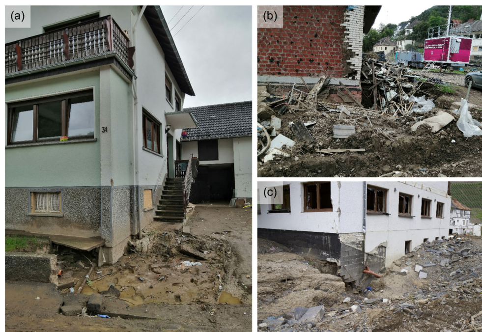
FIGURE 4 Scour at various buildings corners in: (a) Schuld; (b) Altenahr; (c) Marienthal.
