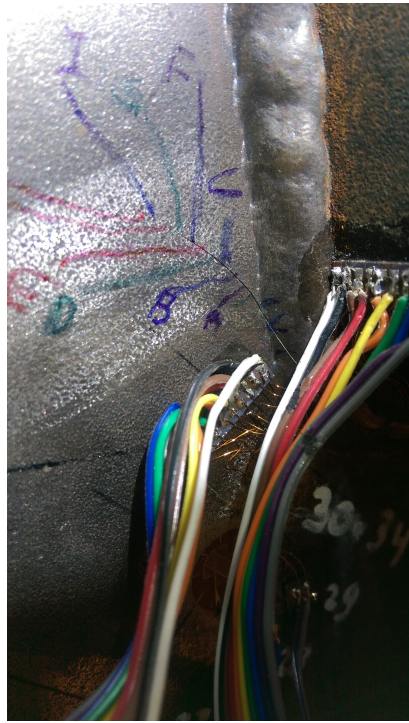
Figure 3.14: Fatigue crack (25 mm) propagating into the crossbeam of the bridge deck
