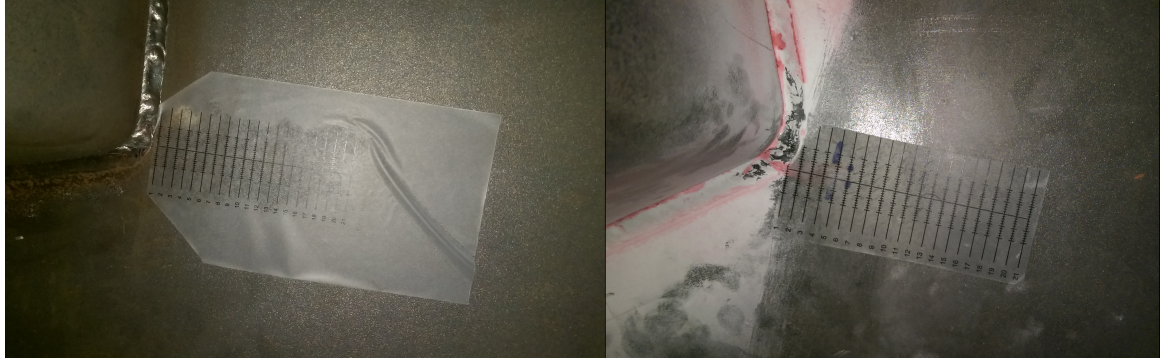
Figure 3.16: Fatigue crack propagating into the crossbeam of the bridge deck
