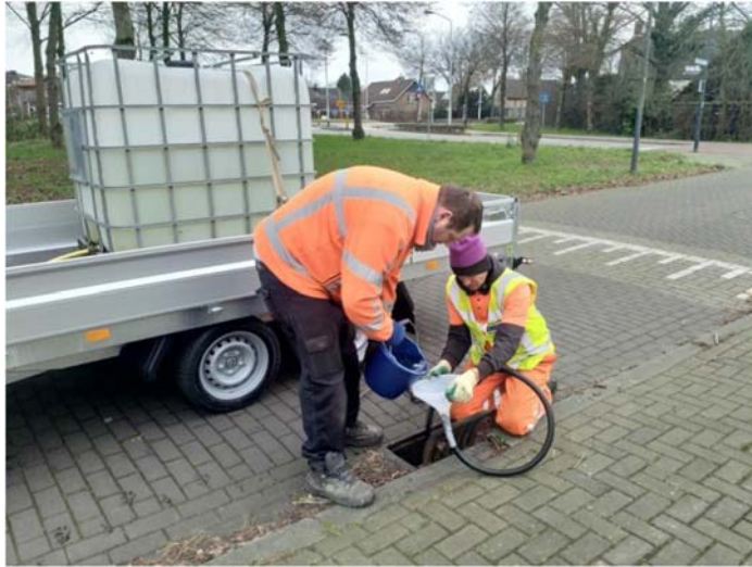
Figure 6.17 Pouring cold water onto the cable, in the underground sewer, using a hose and a funnel for validation of the measured distances by the DTS system. Source: courtesy Remy Schilperoot (Partners4UrbanWater).
