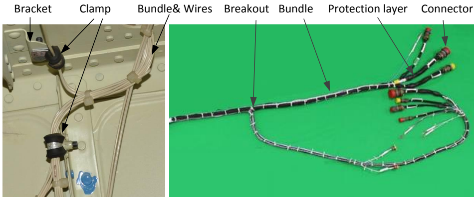
Figure 2-1: A harness installed in an aircraft (left); and a harness with an independent view (right) [18]
