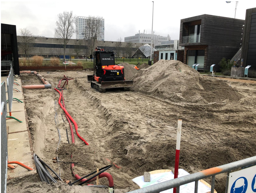
Figure B.1.: Excavation done prior to the construction of the Heat Square for installation of the fibre-optic cable and other required infrastructure.
