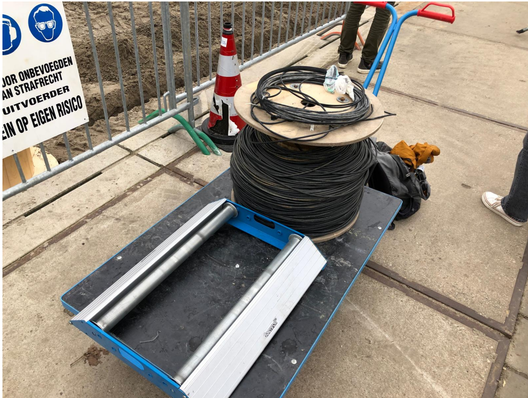
Figure B.2.: Fibre-optic cable coil prior to digging the cable into the ground.
