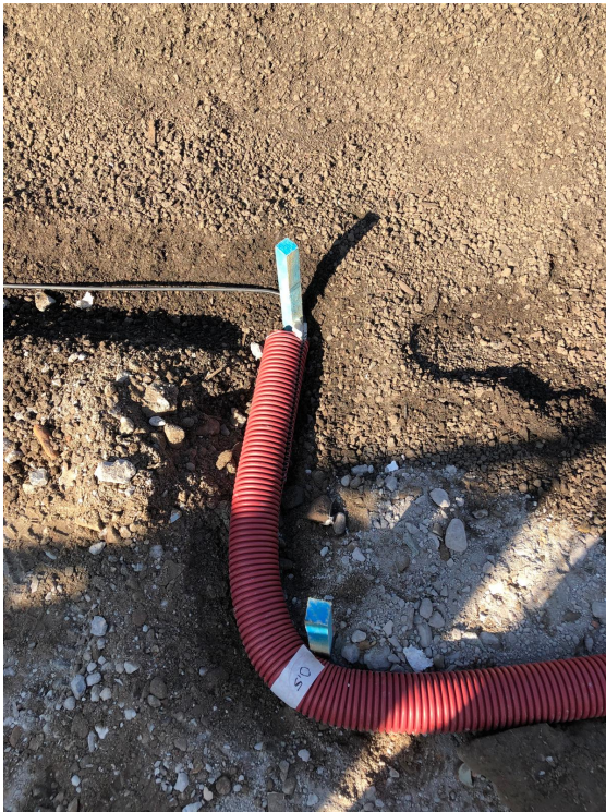
(a) LAF of cable is marked at every turn and change of pipe encasing.
