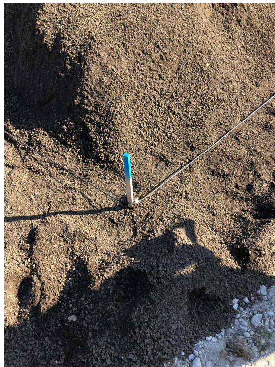
(b) Stakes which mark the turns of the cable path, used for maintaining tension and locating the cable at different depth.
