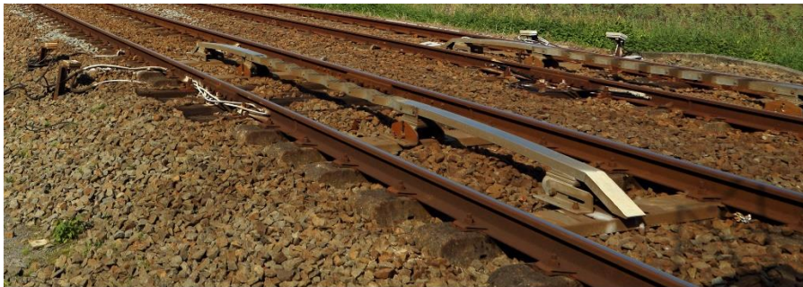
Figure F-3: Crocodile ATP contact, clearly reaching above the top of rails. Marc Ryckaert.
