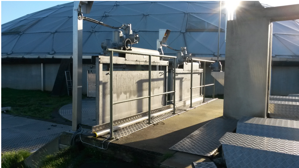
Figure D.2: Picture of the controllable valves to dynamically operate the PCs in the Primary Clarifier Control.
