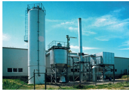
Figure 2: Flue gas cleaning of the HZG brickyard (1997)
