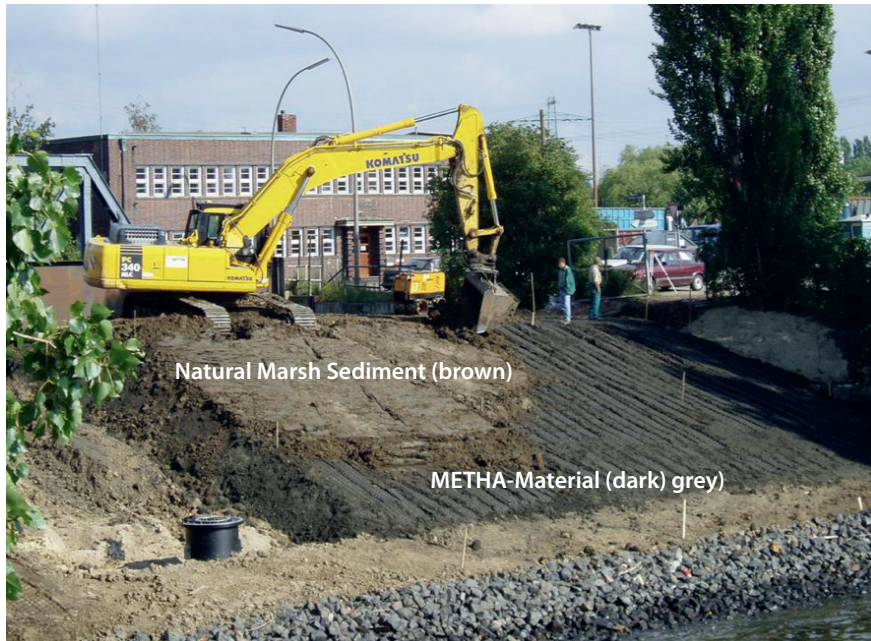
Figure 1: Photo of pilot dike construction using METHA Material below a layer of natural marsh sediment in 2004. Photo by J.Gebert.
