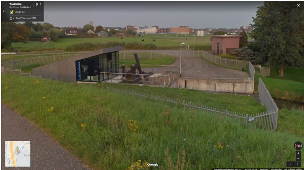
Figure 4-8: Harnaskade pumping station, Delft ( www.google.com/maps accessed: 2018)
