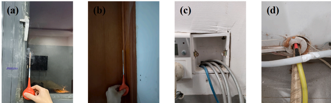
Fig. 5. Approximate detection of air leakage paths: Smoke pen test: (a) Exterior window and (b) Interior door; Direct observation: (c) Socket base and (d) Through-wall pipeline.
