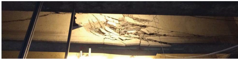
Figure 6. Shear failure of T-girder in test 1. The diaphragm is located on the left side and the end support on the right side.
