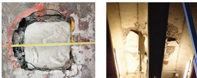
Figure 7. Punching failure of the deck slab in test 1, showing top view and measurements in cm (left) and bottom view (right).
