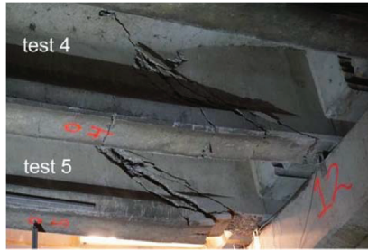
Figure 8. Flexural shear failures in test 4 and 5.
