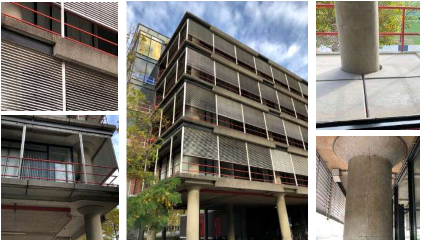
Figure 82. Collage of images of the current state of the concrete elements of Gemini south building.
