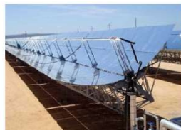
Concentrated solar power
