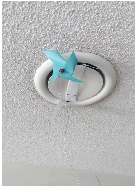
Fig. 73 - The fan is attached to the ceiling supply valve for the two-day evaluation. Residents used to fan to align their actions to system activity
