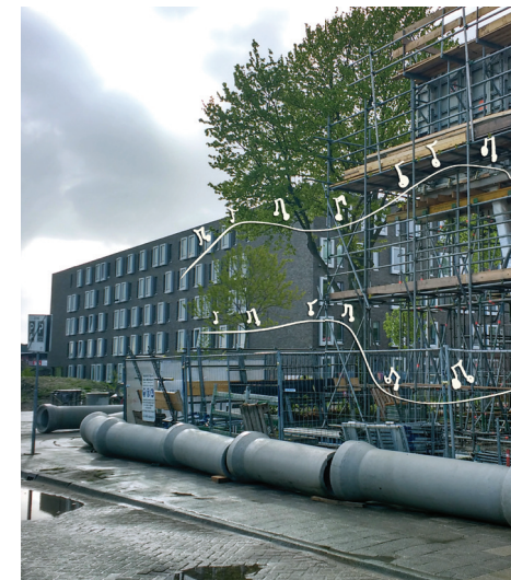
Fig. 25 - The construction work besides the student building made the skill to balance noise and fresh air very relevant.
