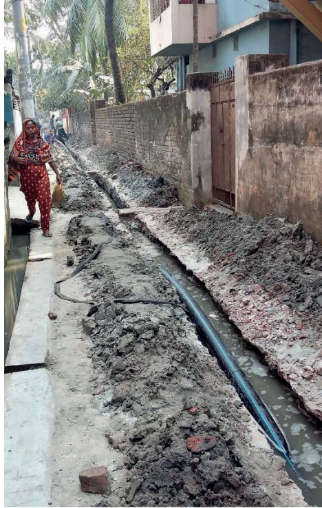
Figure 5.9 Construction activities in Sarkarpara area of Khulna city as part of KWASA's new pipeline project (Photo courtesy Gomes, 2017)
